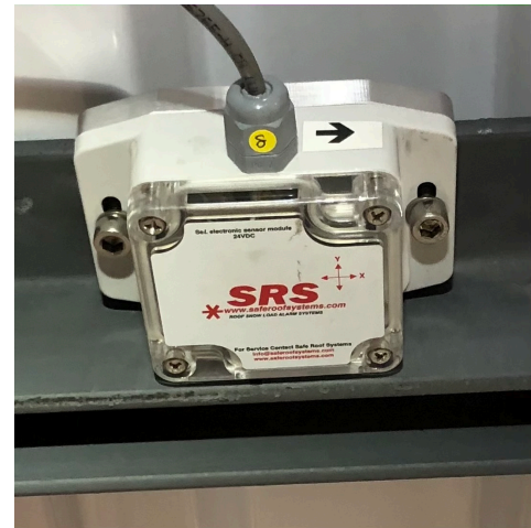
Electronic deflection measurement
